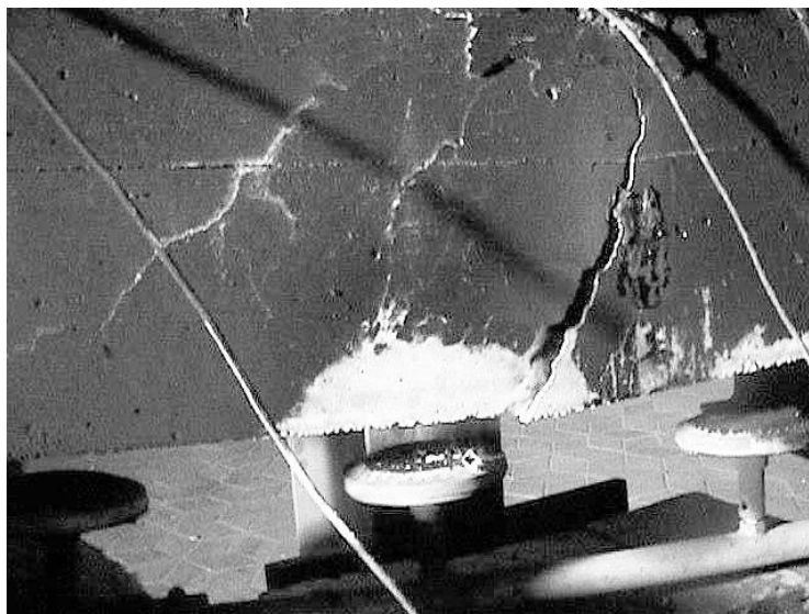
Fig. 8. Fire penetrating cracks in a beam specimen.
