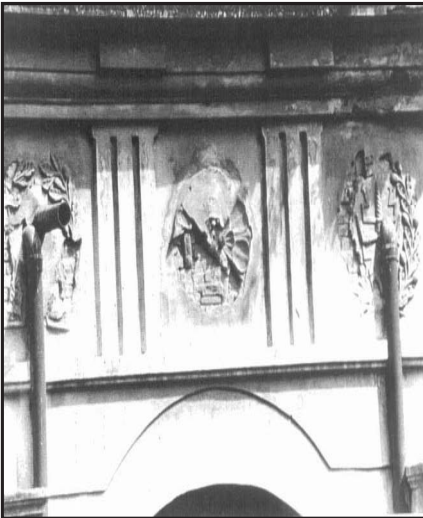
LEAKAGES FROM RAIN WATER PIPES
