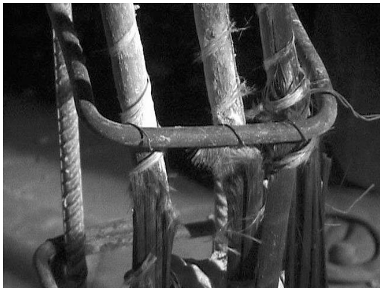
Fig. 10. GFRP bars after fire.
