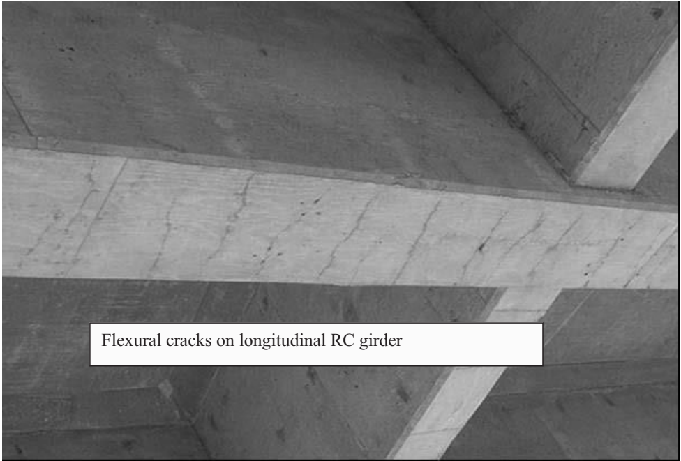
Fig. 13. Flexural cracks on the longitudinal reinforced concrete girders in the Louisa-fort Gay bridge
