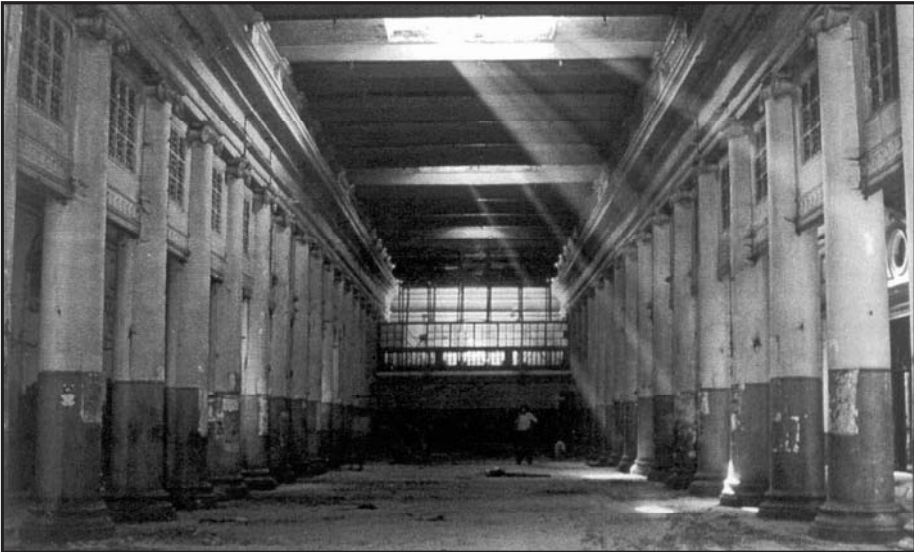
DAMAGED COLUMNS ON FIRST FLOOR
