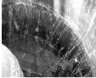
Fig.2b. Water leakage in tower before repair.
