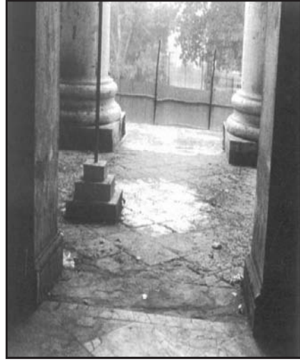
RAIN WATER FALLING ON THE FRONT PORTICO
