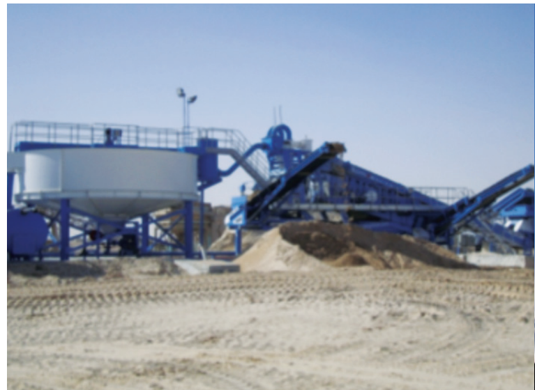
Advance sand washing plant
